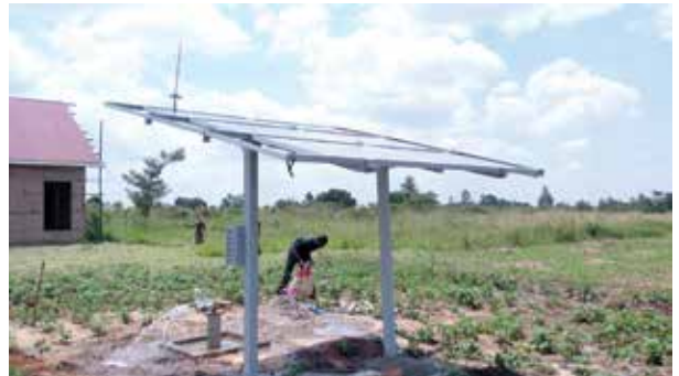
Solar Water Pumping
